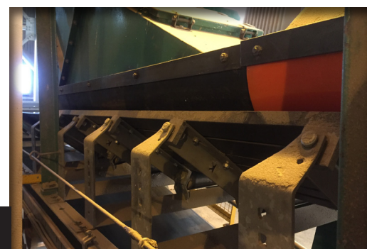
Photo: K-Sure® Belt Support System installed at transfer point.
