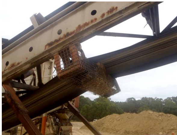
Photos of non-complying steel guards on various sites
