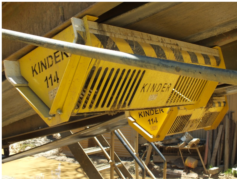
Photo on site of installed K-Protector® Return Idler Guard. 100's of user details available upon request.
